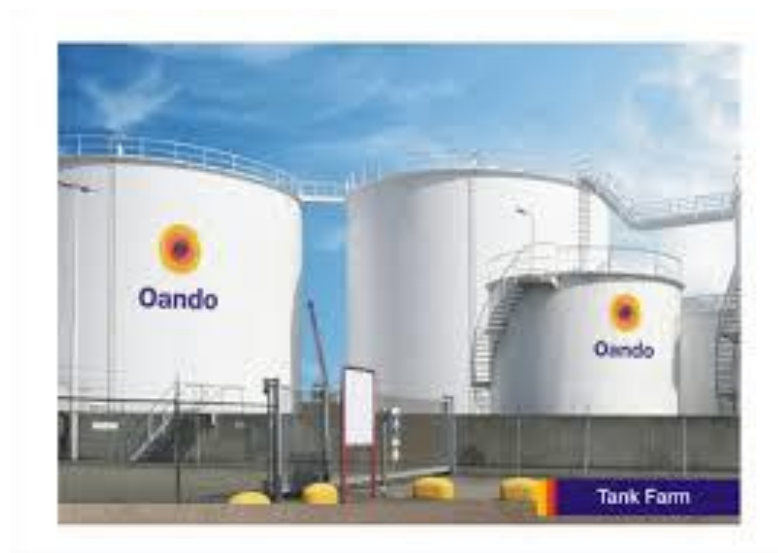
Plate 2.2 : Oil Tank Farm (To the naked eye, no emissions from an oil storage tank are visible, but with the aid of an infrared camera, one can detect CH 4 being emitted).
